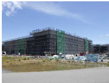
Volume reduction facility (To be completed in 2023)
