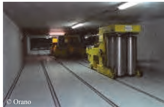
ECC is a fully remote and automated facility in Orano La Hague where hundreds CSD-C are temporarily stored in a safe and organized way, until final disposal site is available.
