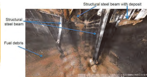
Example of types of waste identified inside the PCV on TEPCO picture
